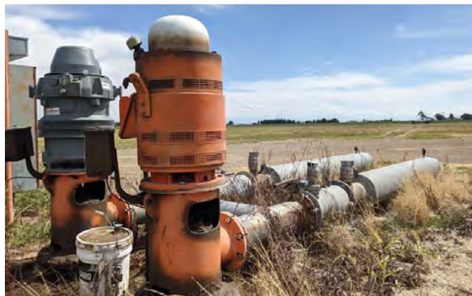
A groundwater pump seen in the San Luis Valley, Colorado. Groundwater overdraft has become a serious issue across the western US in recent years and could be improved with increased monitoring.
